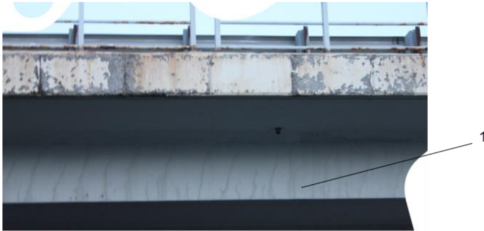
Fig. 1. Normal bending cracks (1) in reinforced concrete bridge beams (Uman, Ukraine)
